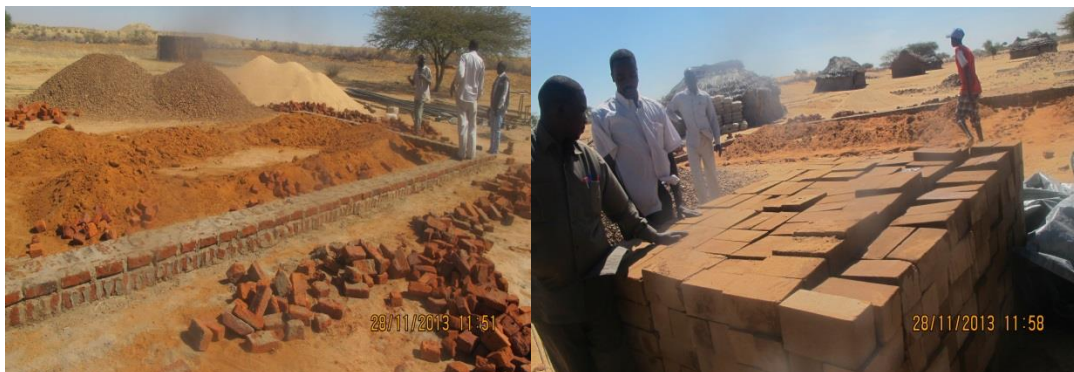
2 classrooms construction (foundation work) in Umkadoia West Basic School and SSBs production to be constructed with.
